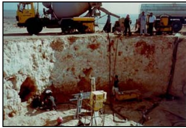
Fig-1: Cavity Probing and Pressure Grouting works for a site in Al-Hufoof
