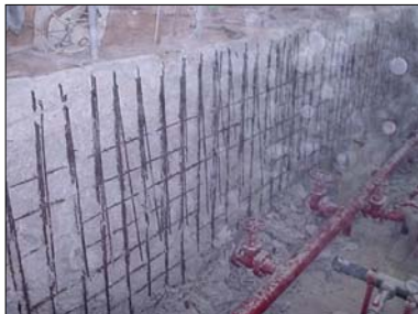
Water tank wall damaged by Corrosion
