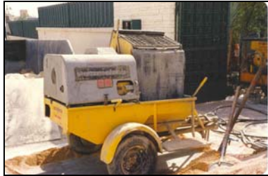
Fig-5: Grouting Pump & Mixer
